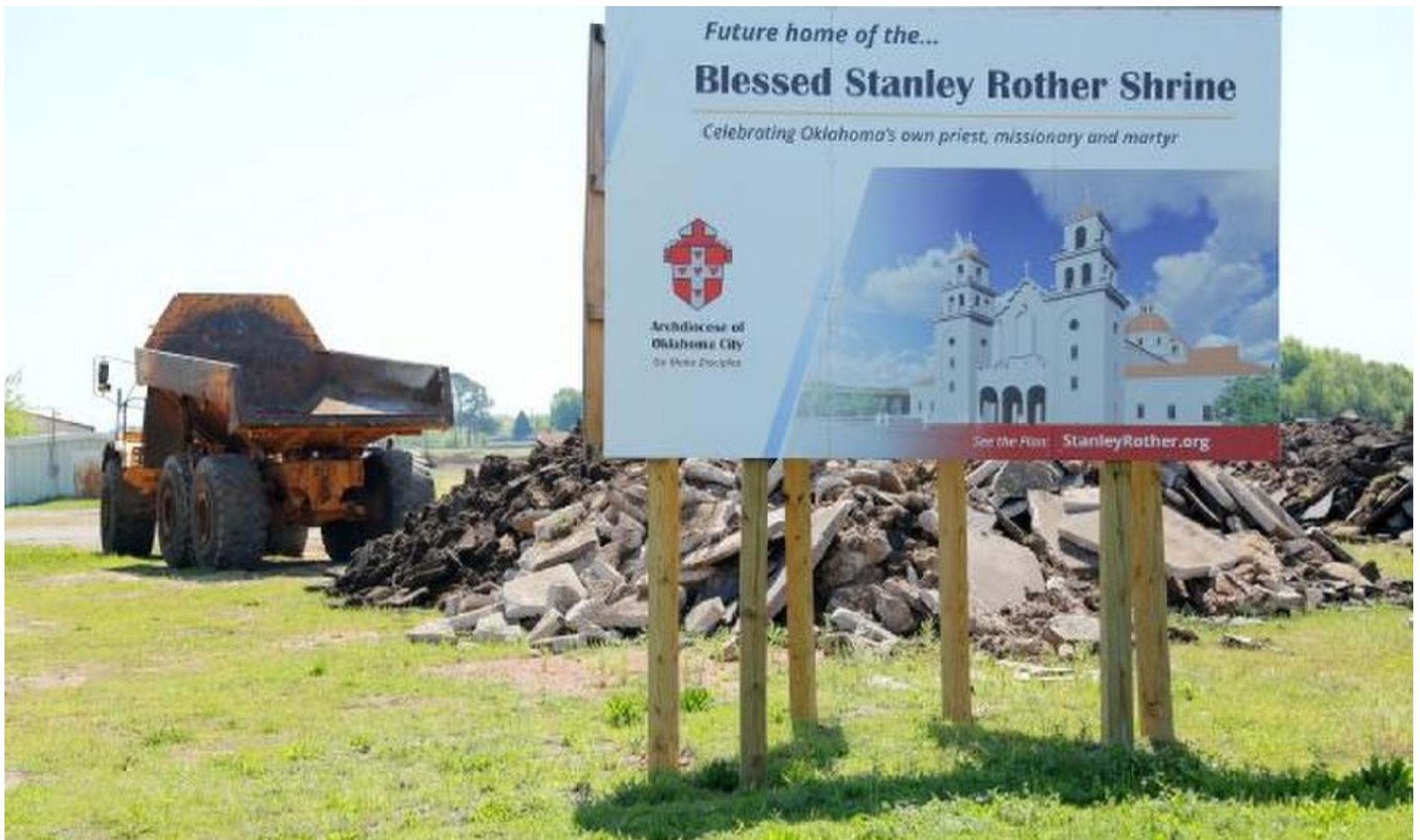
In this April 21 photo, excavation work begins at the construction site for the Blessed Stanley Rother Shrine on SE 89, between Shields Boulevard and Interstate 35 in Oklahoma City. [Doug Hoke/The Oklahoman]
