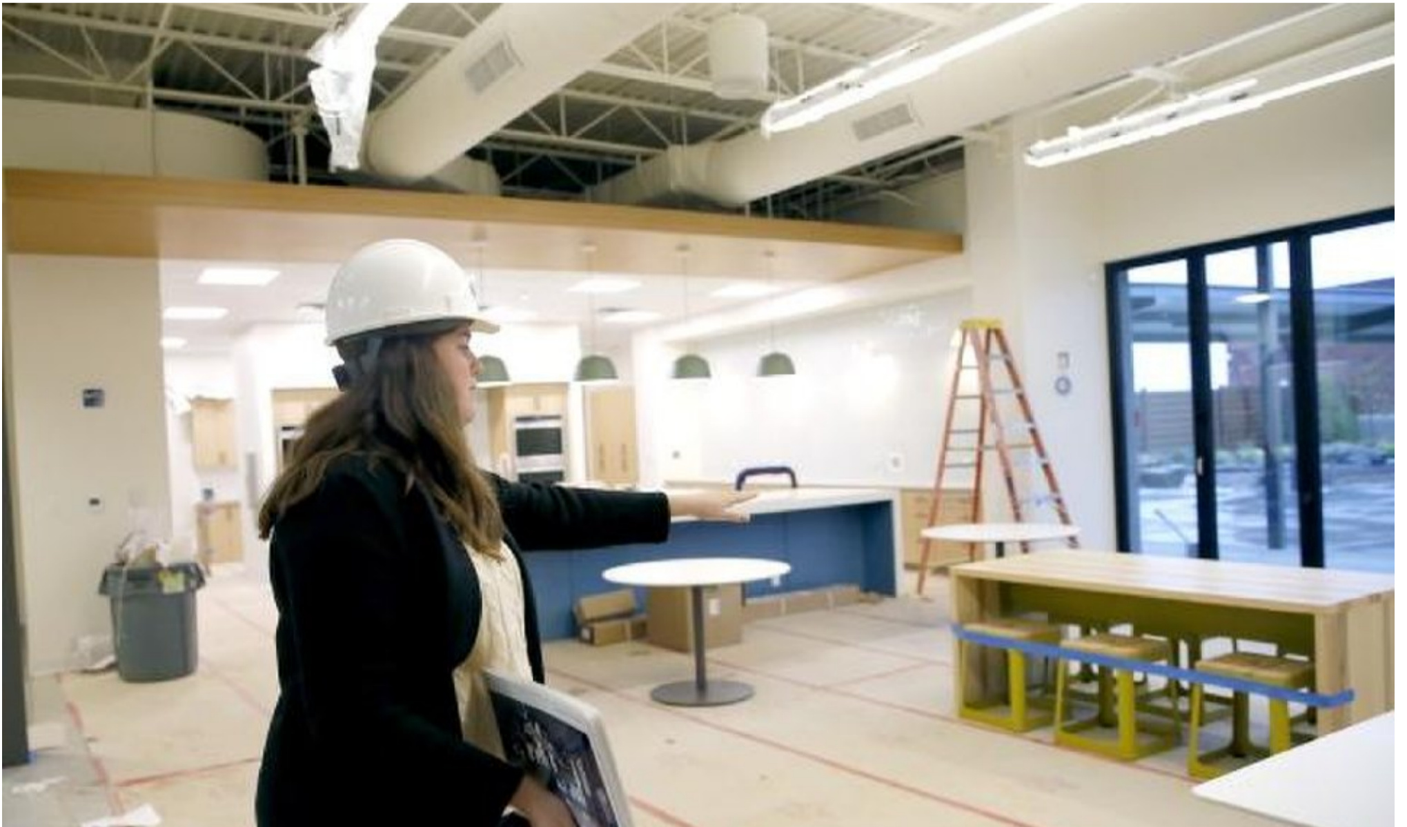
Rose Faherty shows the kitchen area at the new ReMerge building at 823 N Villa. [Sarah Phipps/The Oklahoman]
